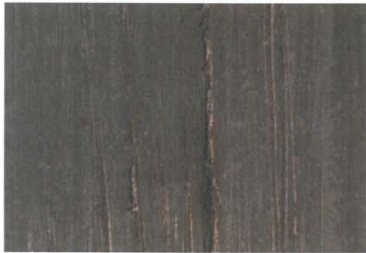
Fig. A.3 Inner wall surface; wear tracks in the length direction of the pipe (shown surface: ca. 10x10 mm).
